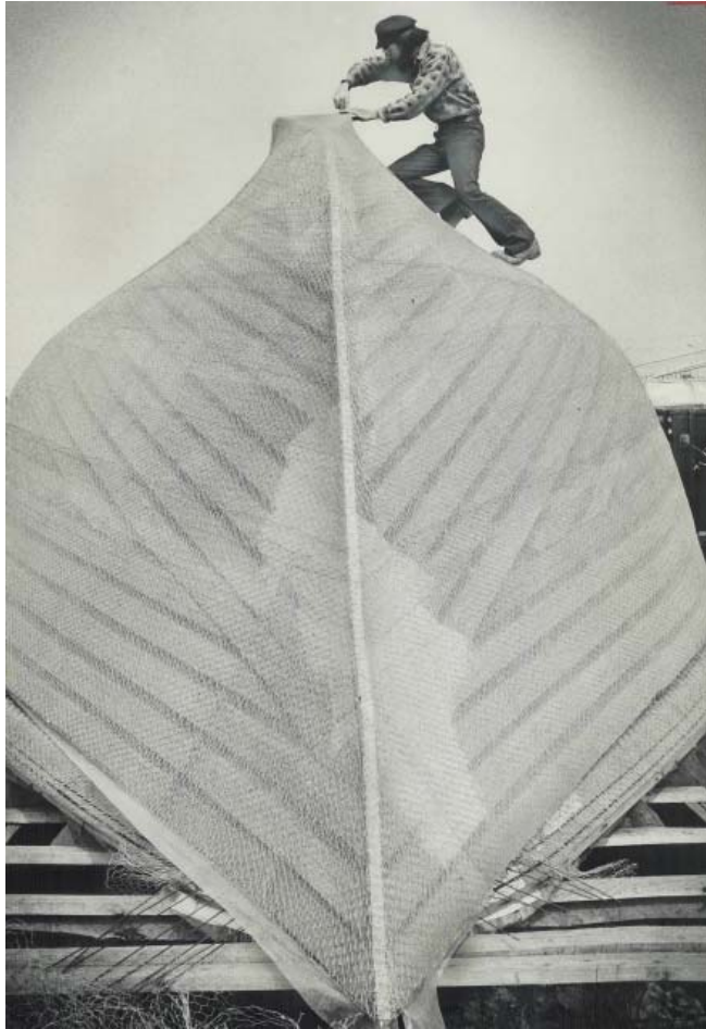
1975 : Warren lays the steel mesh hull of Solstice Moon. photo credit: Boris Supremo, Toronto Star Archive, Toronto Reference Library
